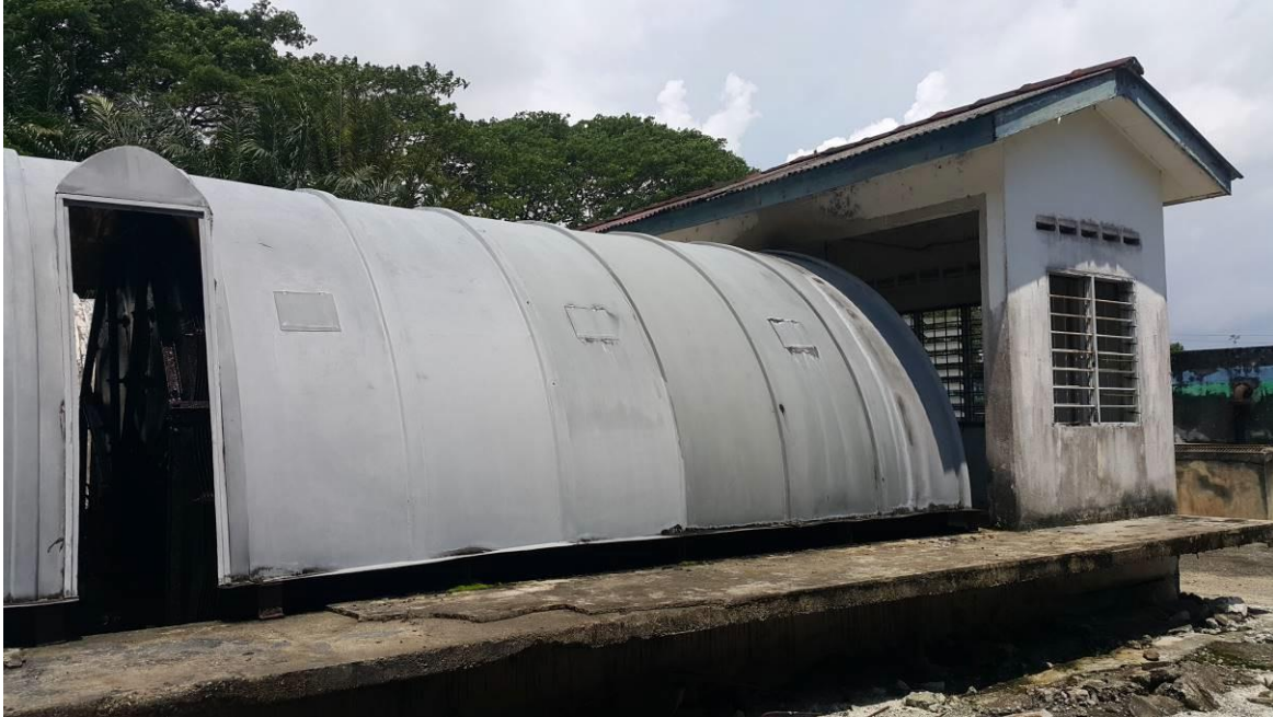
RBC ROTORS IN CONCRETE TANKS IN MALAYSIA US MADE - GRP COVER
